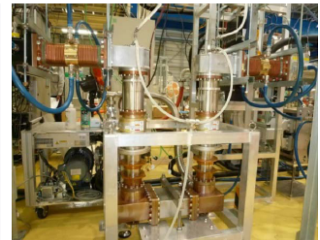
High power test stand
