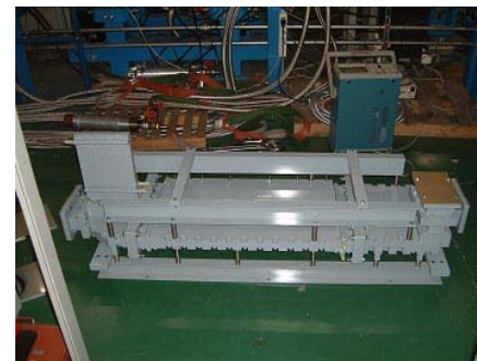
1.3GHz CW 40kW Isolator (JAEA)
