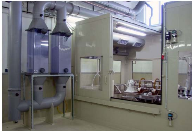
Electropolishing plant for XFEL cavities
