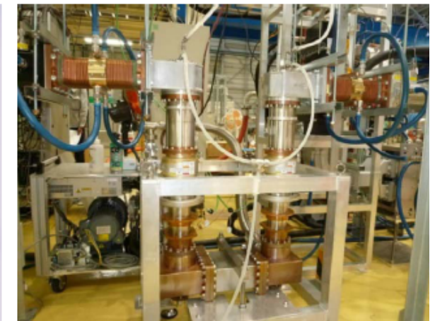
High power test stand
