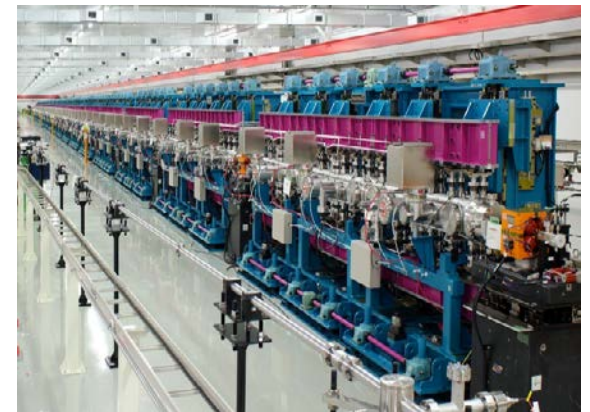
In-vacuum undulator to produce SASE FEL
