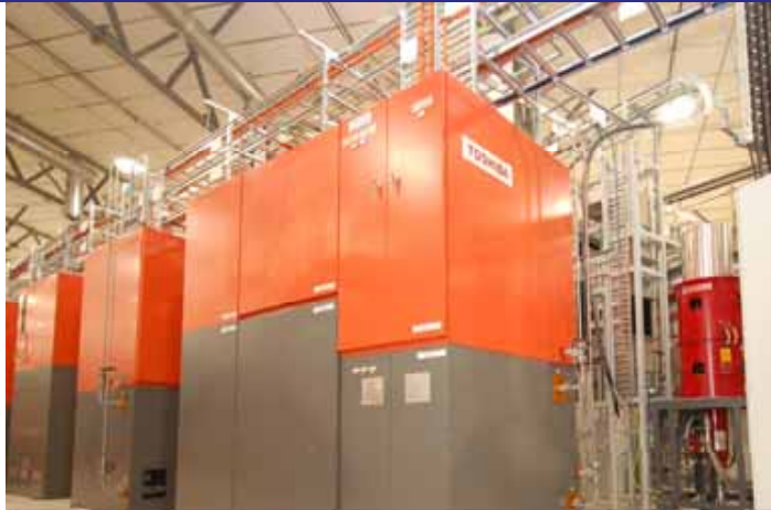
RF Power Supply & Klystron
