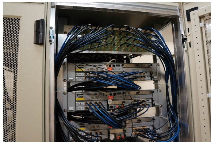
Figure 5: A part of the new beam position circuits installed into the standard rack.
