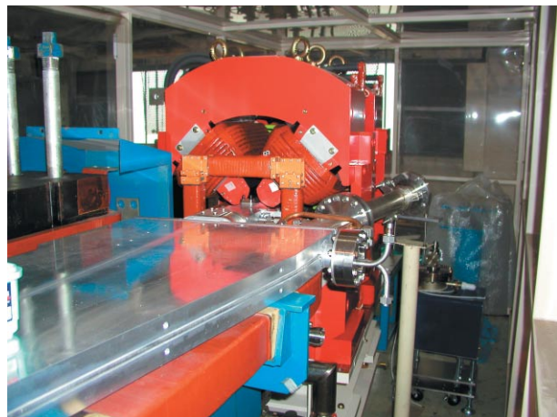
Figure 9 Photograph of the test bench installed in the power supply building.
