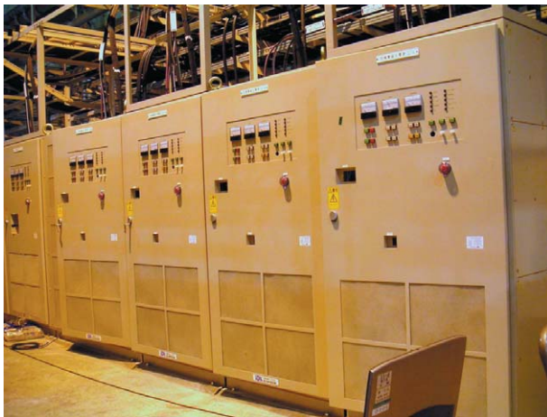
Figure 18 Photograph of the power supplies.
