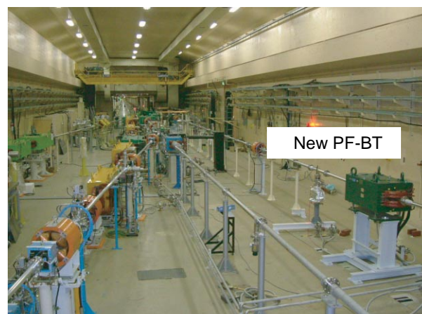
Figure 15 View of the new PF-BT.
