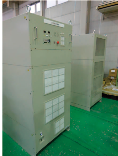
Figure 3 SXF and SXD power supplies in the factory.
