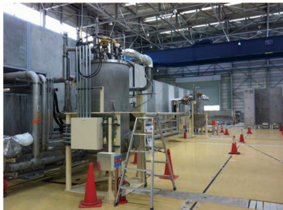
Figure 25 2K helium refrigerator cold box for the main linac under cold test.
