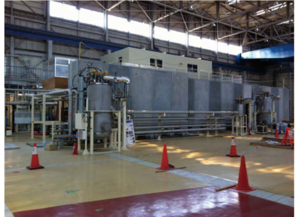
Figure 23 2K helium refrigerator cold boxes which will be connected with cryomodules of superconducting RF cavities for injector and main linacs.
