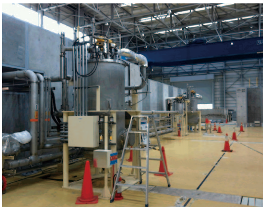
Figure 11: 2K refrigerator cold boxes and transfer lines for cryomodules.
