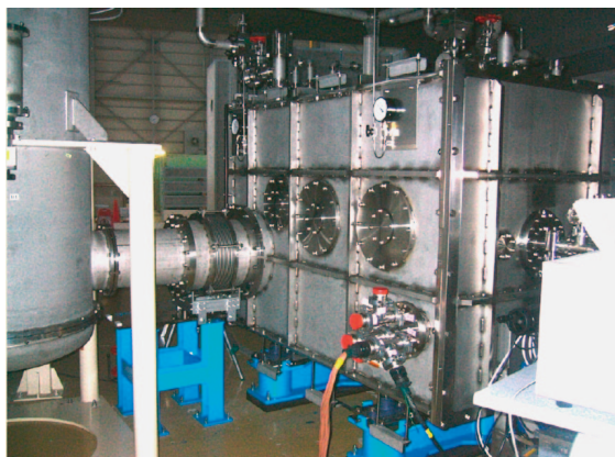
Figure 5: Completed cERL injector cryomodule installed in beam line and connected with cold box.
