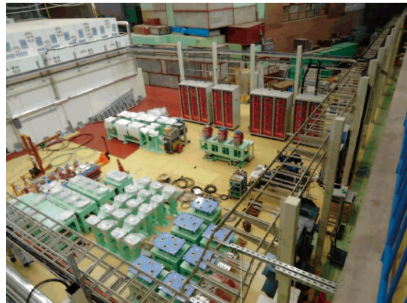
Figure 13: The girders and power supplies at the ERL Hall.
