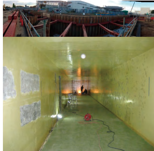
Figure 4: Upper photograph: the precursor tunnel in November 2013. Lower photograph: the inside of the tunnel before painting.
