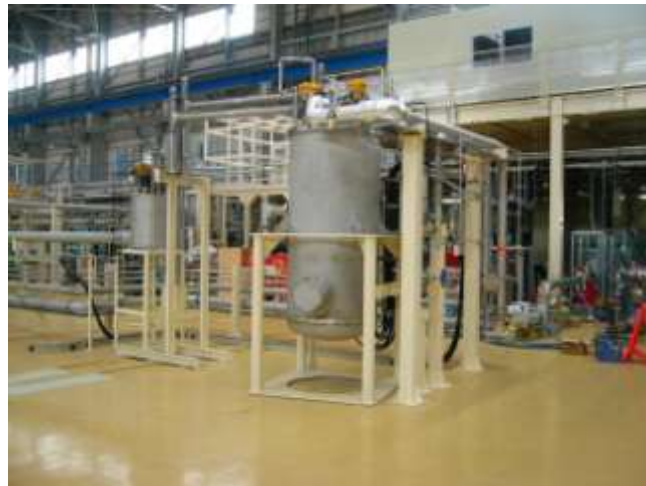
2K cold box and end box
