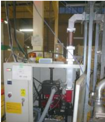
30kW CW IOT for main SCC
