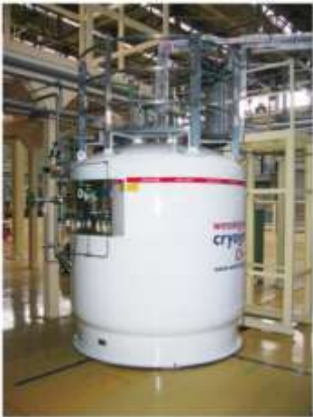
3000L liquefied helium storage vessel
